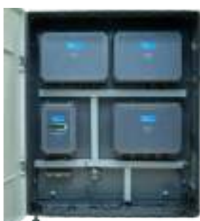
Interior View of xMasm10 - Wired Solution
