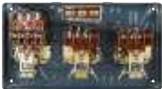
Interior View of MK2 SASD
