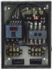
Interior View of MD Starter+ DOL Starter
